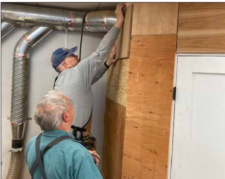
Don Cooke in the back and Bob Reinhardt installing the final piece of sheathing to the enclosure.
