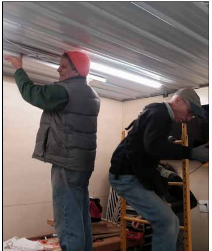
Mike Guiliano and Andy Moss install spacers on the metal ceiling to anchor the pipes
