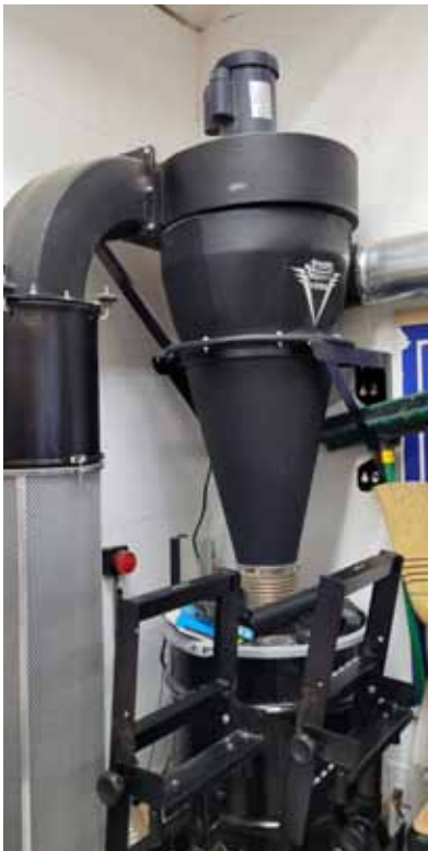
Paul's dust collector system
